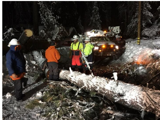
Fallen trees during the 2017 winter storms were responsible for many downed power lines and were time-intensive to remove and repair.
